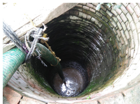
Condition of the well before cleaning
