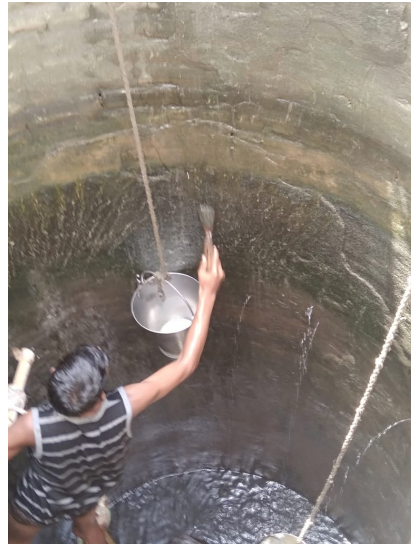
scratching green rigid algae from the inner wall
