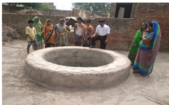
condition of the well before cleaning
